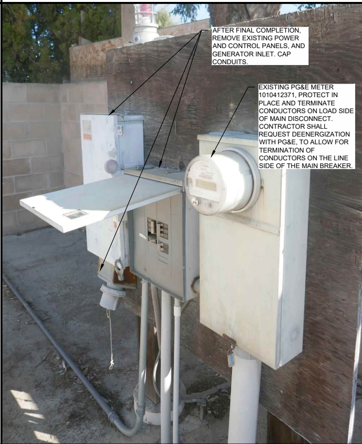
7 EXISTING PG&E METER AND POWER AND CONTROL PANELS E400 NOT TO SCALE
