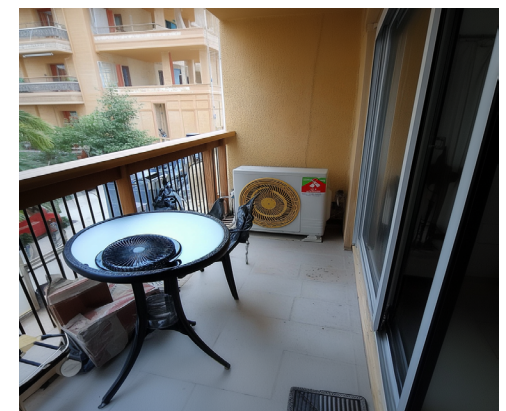
✗ Air conditioning condenser exposed to view without screen.
