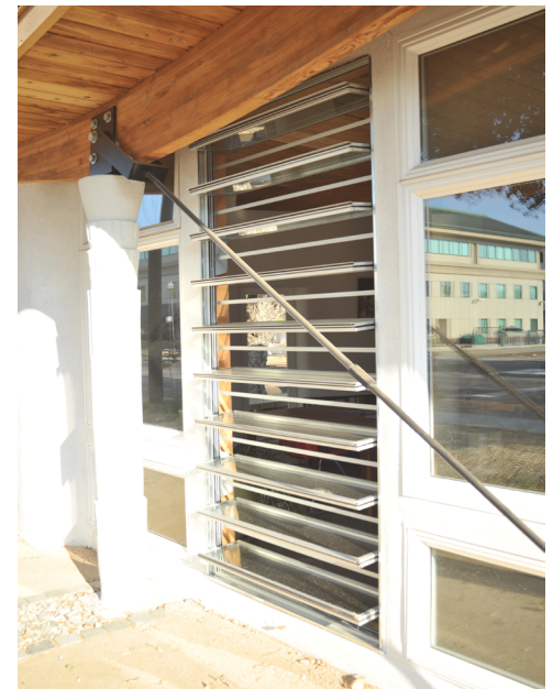
+ Nighttime ventilation louvers.
